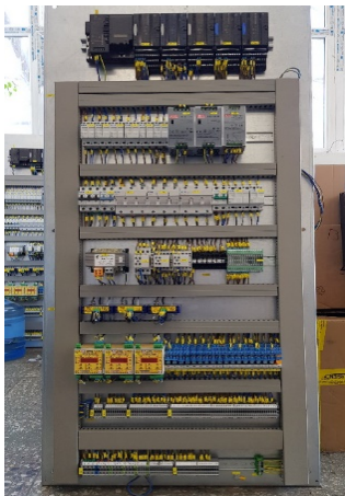
Fig. 1 – Automation cabinet for a piston compressor at Bustuchin station.
