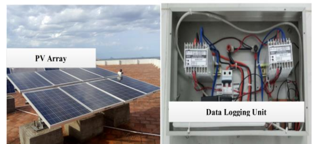
Fig. 4 – Solar PV array and its data logging unit.
