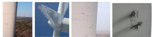
Fig. 2 – Sample images of cracked wind blade images.
