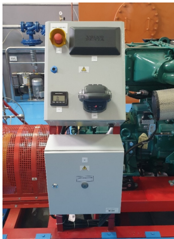
Fig. 7 – Engine local control point console.
