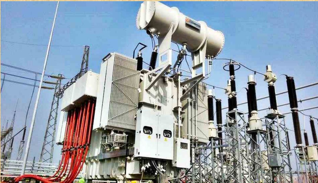
Step-down trafo 73 MVA 110/15/6.6 kV; 15 kV cable output for Saudi Arabia
