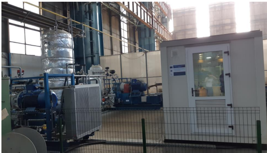
Fig. 1. ROCAES installation with automation and control room
