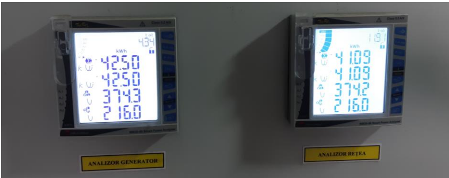
Fig. 3. Power analysers displaying the generated power (left) and power supplied to grid (right)
